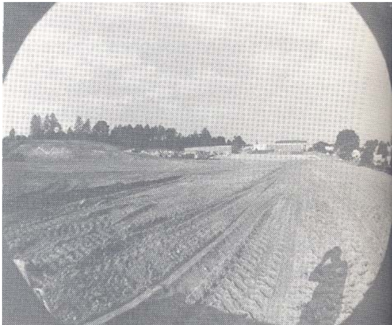
The grading for the parking lot is shown here under way in 1969.
